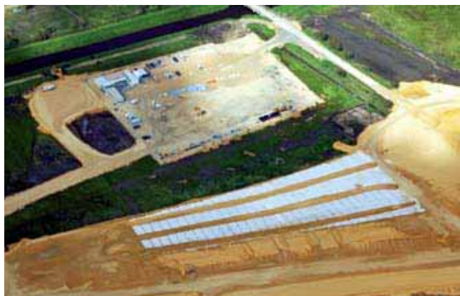
An aerial view of geofabric membrane laid at the Karnup Road interchange constructed as part of NPBH.
